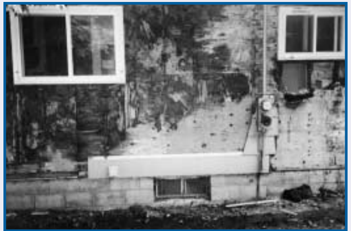
Example of major damage due to excessive build up of moisture.
