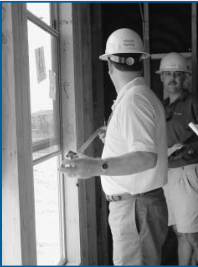
Builders making a quality assurance check on a construction site in Phoenix, Arizona.
